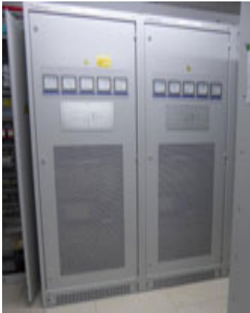
Figure 3: Visual image taken showing mesh in the door of an electrical cabinet
