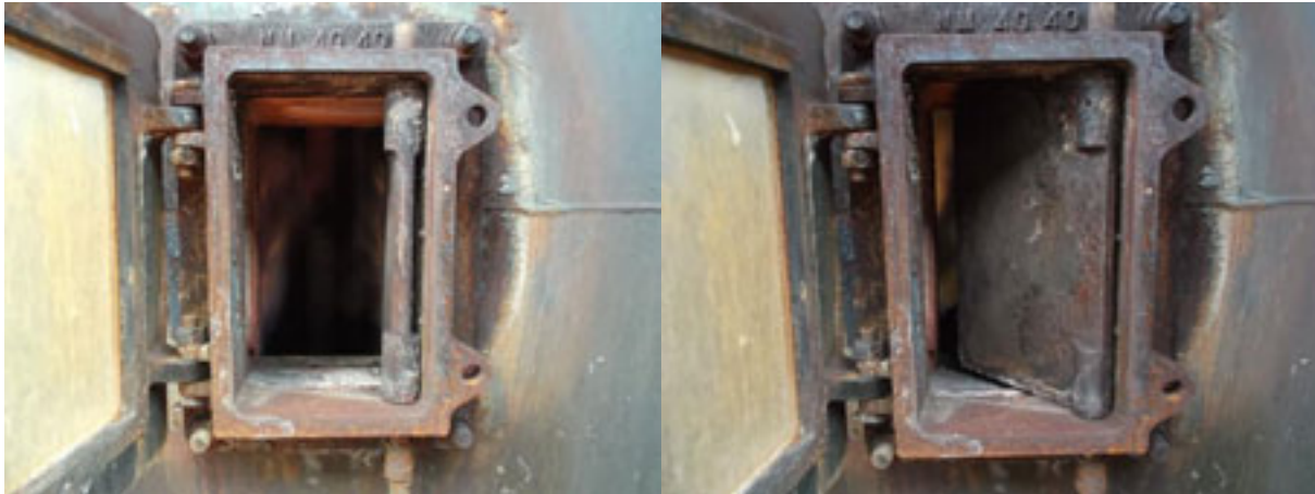
Figure 14: Furnace peephole at maximum and minimum opening
